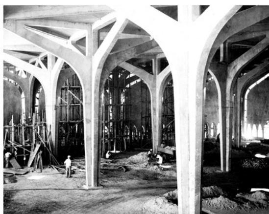
Figure 5: The interior of Dhahran Civil Air Terminal during construction circa 1960. (Source: U.S. Army Photo, courtesy of the Office of History, HQ, U.S. Army Corps of Engineers. OCLC #992716736, Contentdm #509.)
