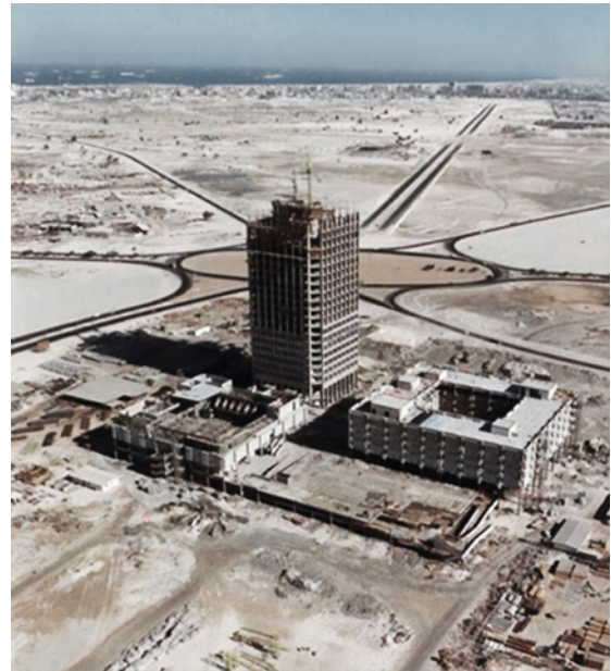
Figure 20: Construction of Sheikh Rashid Tower (Dubai World Trade Center), Dubai 1964. (Source: www.reckontalk.com.)
