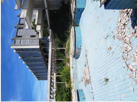
Image 4: Haludovo Palace Hotel. ruin as seen from the pool area, 2011. (Source: Thorsten Schrotterster @Creative Commons Attribution-Share Alike 4.0, Wikimedia.)
